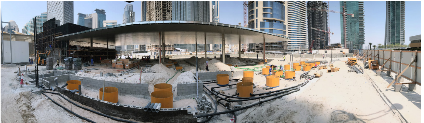
One of over 20 forecourt sites built during the first stage of the project
