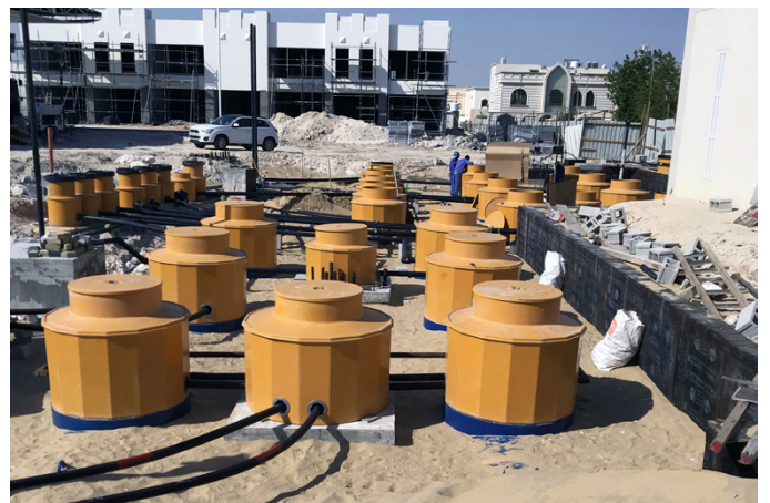
Robust installer training was provided by OPW, including onsite support
