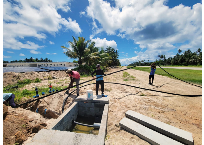
Crossing the runway of the Seychelles island to connect the refuelling pipeline.
