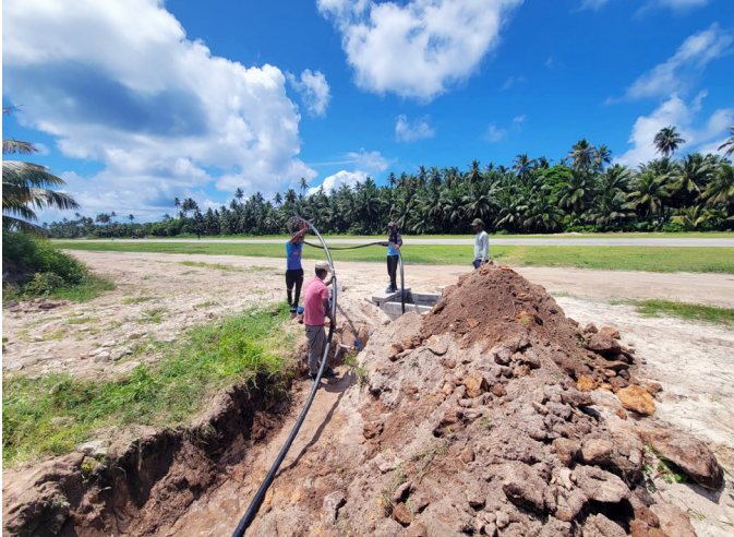
Preparing KPS piping to be installed in a trench in the Seychelles.
