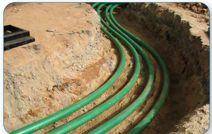
Coiled pipe laid in slight curves that allow the pipes to adjust to temperature changes or ground movement.
