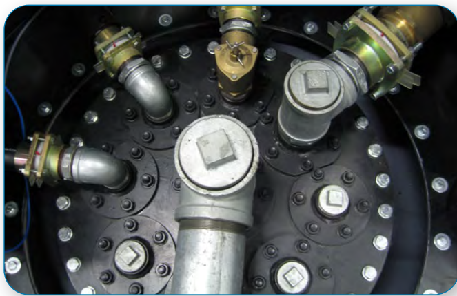
Tank lid connections with flange fittings and shut-off valves.
