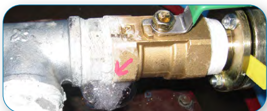
The formation of bubbles is a sure indication of leakage.
